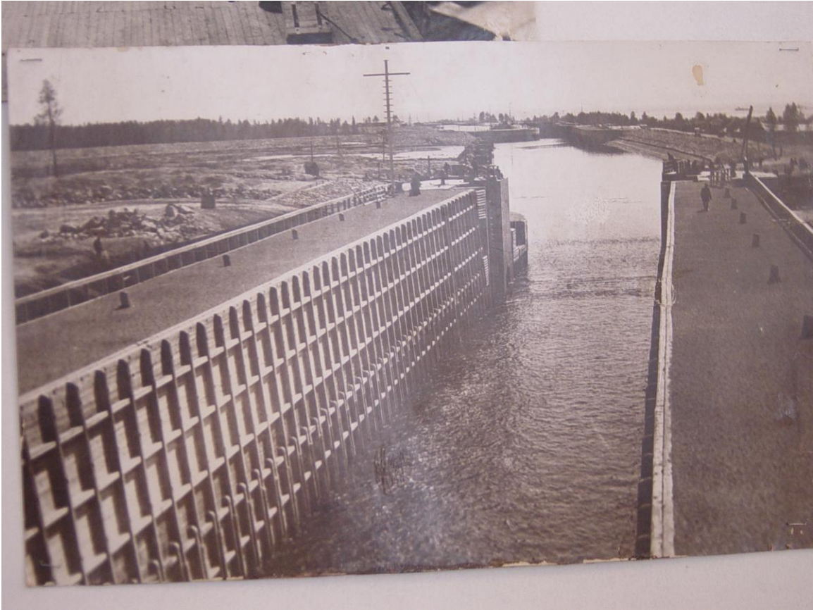
This is one of the 19 locks under construction, made of wood, instead of concrete or iron.
