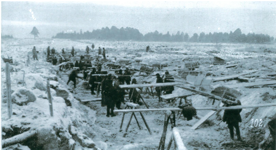
The canal required the digging of a sloping trench 12 feet deep at the center and 141 miles long, much of it through heavy swampland and sheer granite.
